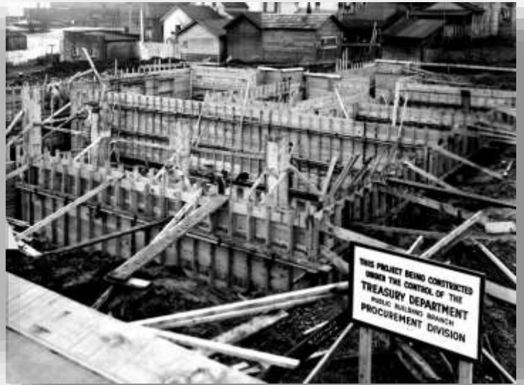
Construction of old Snohomish Post Office c.1937 (sign reads: This project being constructed under the control of the TREASURY DEPARTMENT public building branch PROCUREMENT DIVISION)
